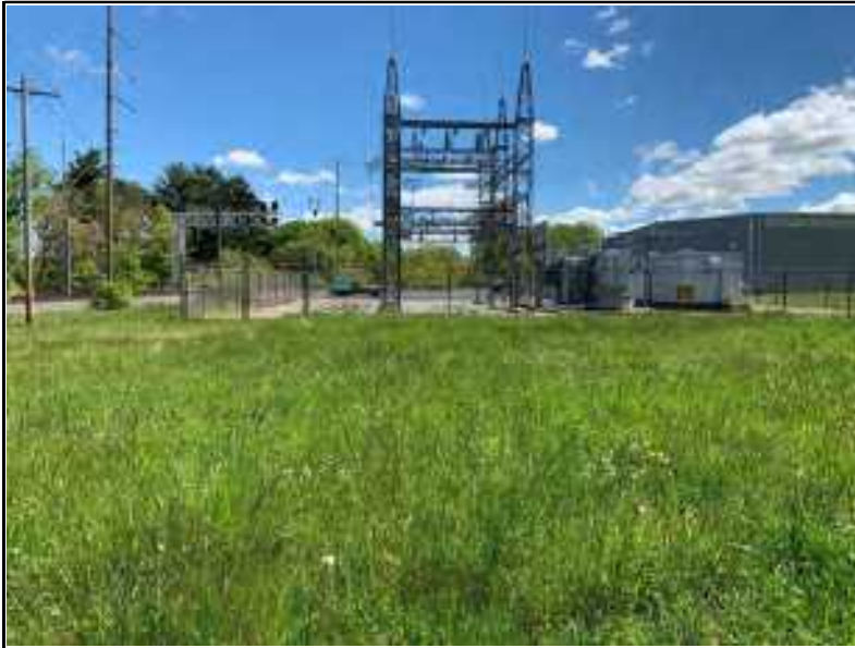
Photo-31 From the northwestern corner of City of Amherst property toward the existing substation
