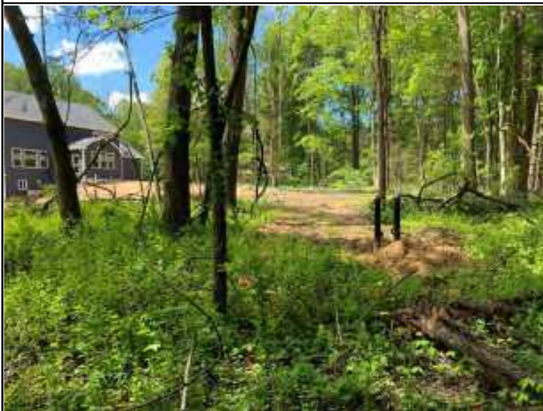
Photo-24 From LS09 towards newly constructed house and installed underground utilities at southern edge of ROW
